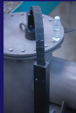
Pump Cable Tray (HDPE casing)
