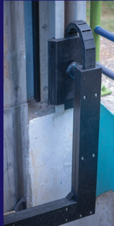
Electrical Cable Tray (HDPE casing)
